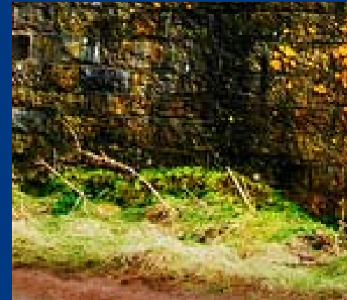
Earth butting against a wall can cause rising damp
