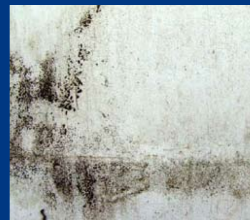
Penetrating damp is often caused by problems with the plumbing
