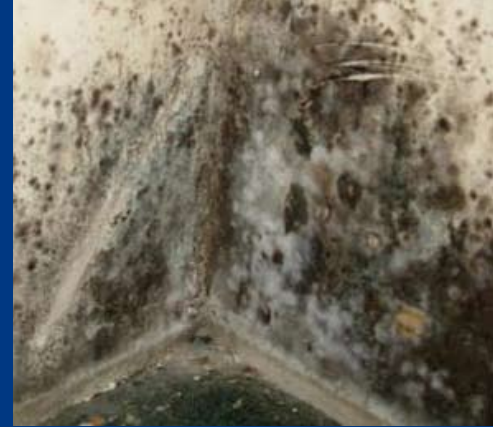
Mould is often present when damp is caused by condensation
