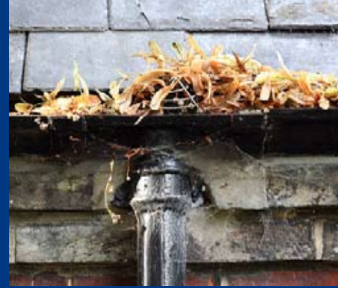
A blocked gutter can cause penetrating damp
