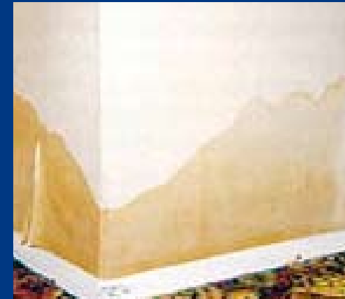
Clear water marks rising from the floor are evidence of rising damp
